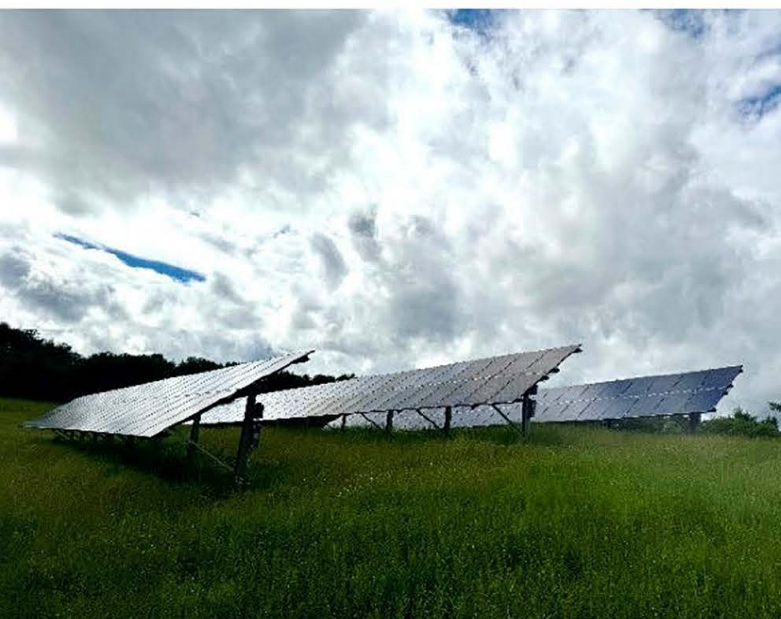
Planson HQ: On-campus solar arrays
