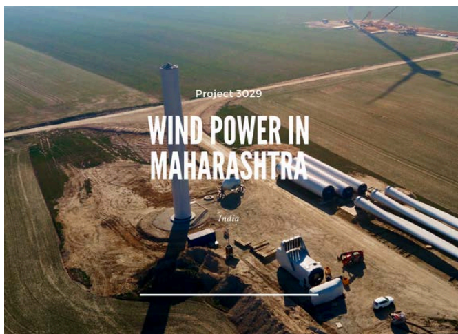
Project 3029: Wind Power in Maharashtra
