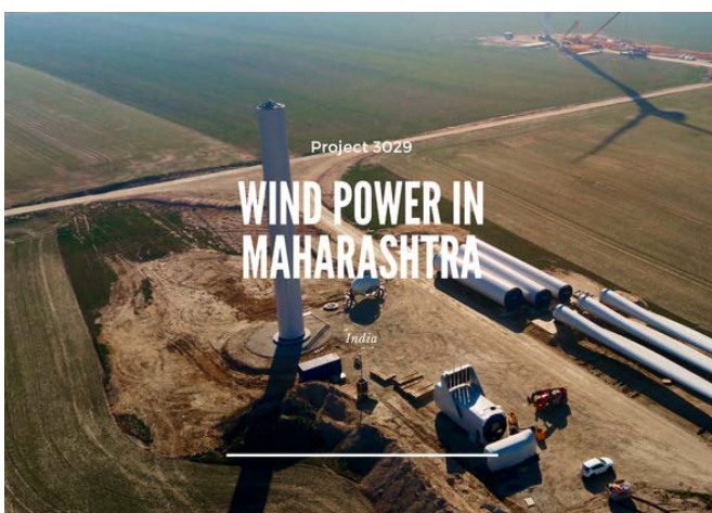
Project 3029: Wind Power in Maharashtra
