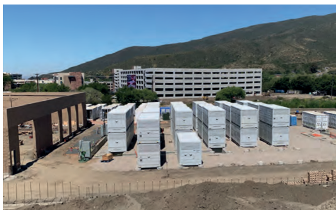
Invinity's 10 MWh VFB at the Viejas Casino & Resort, the largest VFB in the U.S. – May 2024
